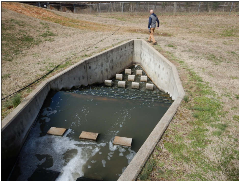
Photograph 8. Cascade post-aeration channel.
